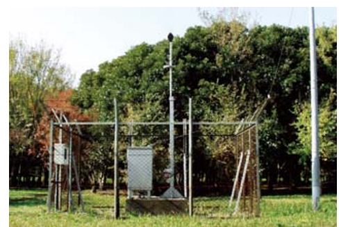
Monitoring system installed in the vicinity of an airport
