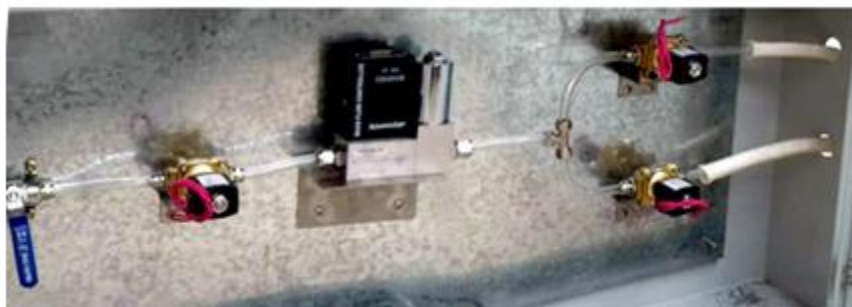
Gas Control Cabinet
