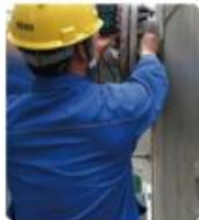
500°C Steam Pipe
